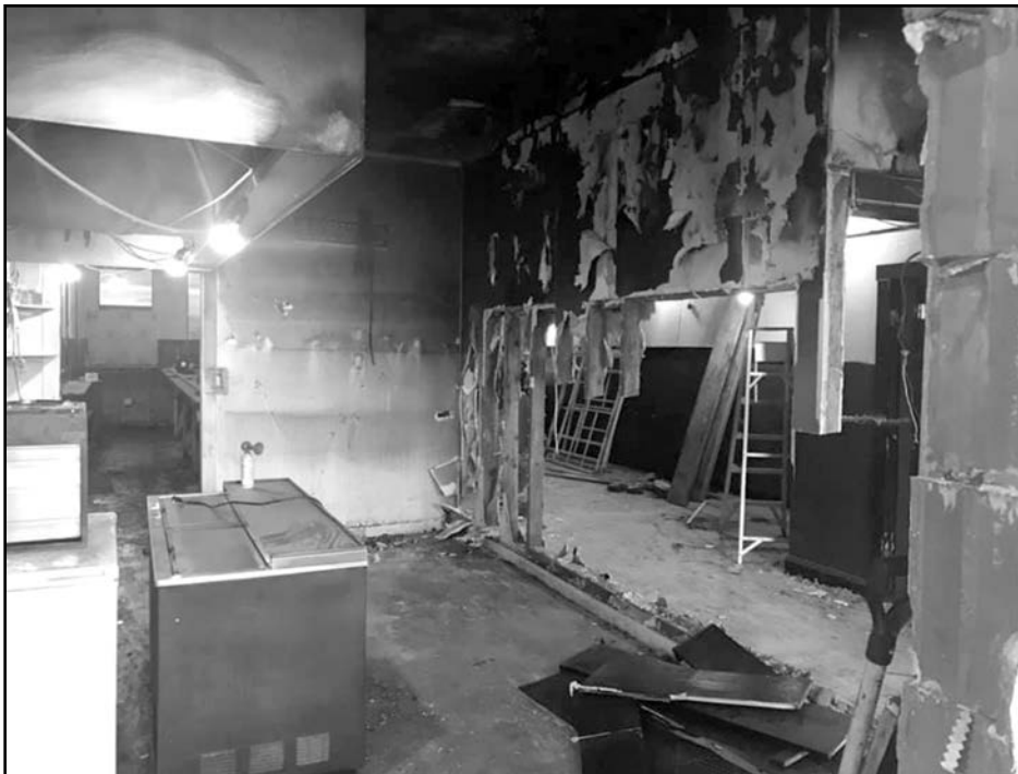
Image of the damage done from the September fire inside the Third Base Sports Bar and Grille on Virginia Avenue in Petersburg.
