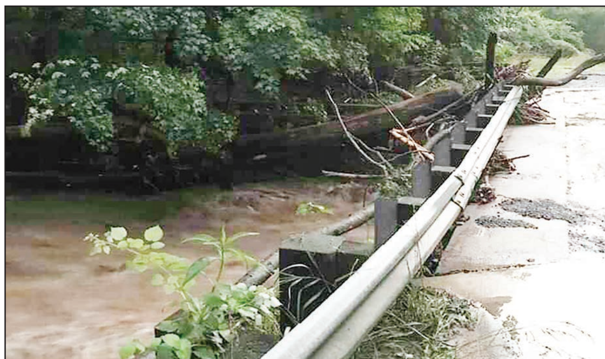
Road damage at the intersection of Keplinger Road and Klines Gap Road.
